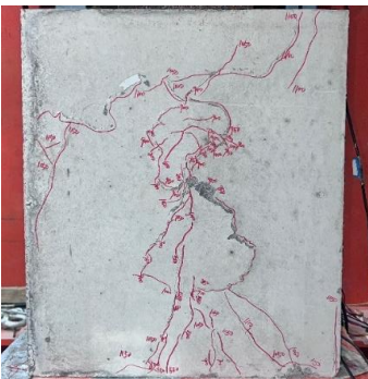
(a) P-C-16-40-10 before destruction
