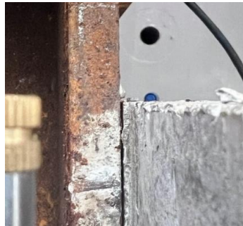
(f) P-C-12-40-10 separation of steel beams and concrete
