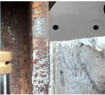
(e) P-E-12-40-10 separation of steel beams and concrete
