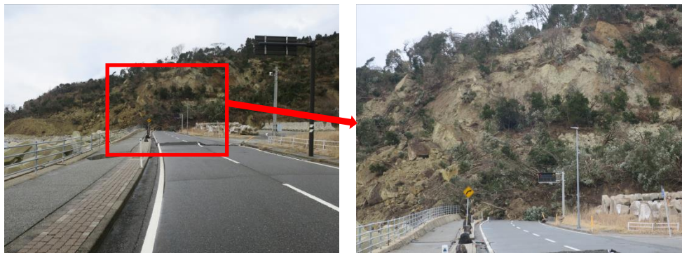
Figure 11. Suzu Maura (slope collapse at the west side of the Osaka tunnel)
