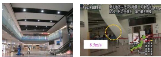
Figure 3. Seismic damage of entrance hall of airport. (Japan earthquake in 2011)
