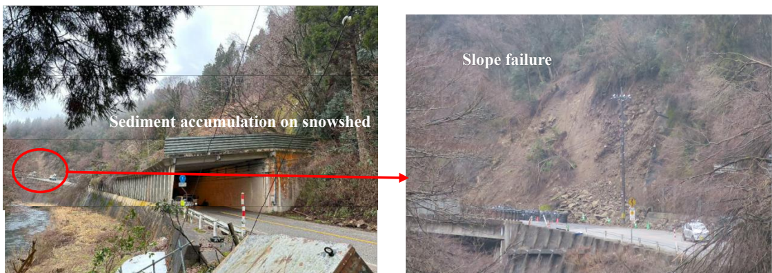
Figure16. Sediment accumulation on snowshed and slopefailure (Wajima Mii Motoe )
