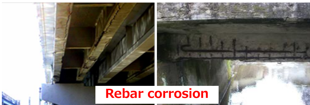
Figure 1. Corrosion of reinforcing steel in the structure
